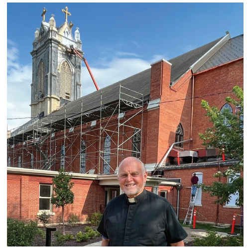
Fr. Dan Knepper stands between the Cathedral Rectory and the Cathedral, with the tower visible in the background. The gray portions are what Fr. Dan explains further on in the article - the tower of the Cathedral is actually sheet metal, which is being repaired and then repainted to once again match the limestone that makes up the rest of the Cathedral tower.
